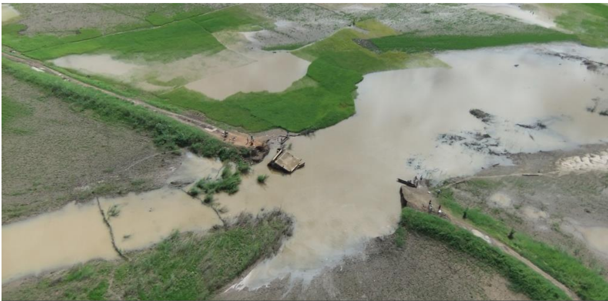
Figure 13 – Collapsed Bridge and Breach at Naminane
