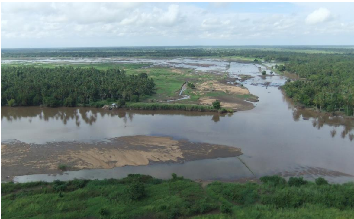
Figure 17 – Intabo Intake Station, Canal and Breach
